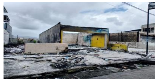
Figure 1. Post-fire business unit in Poka Village (roundabout)
